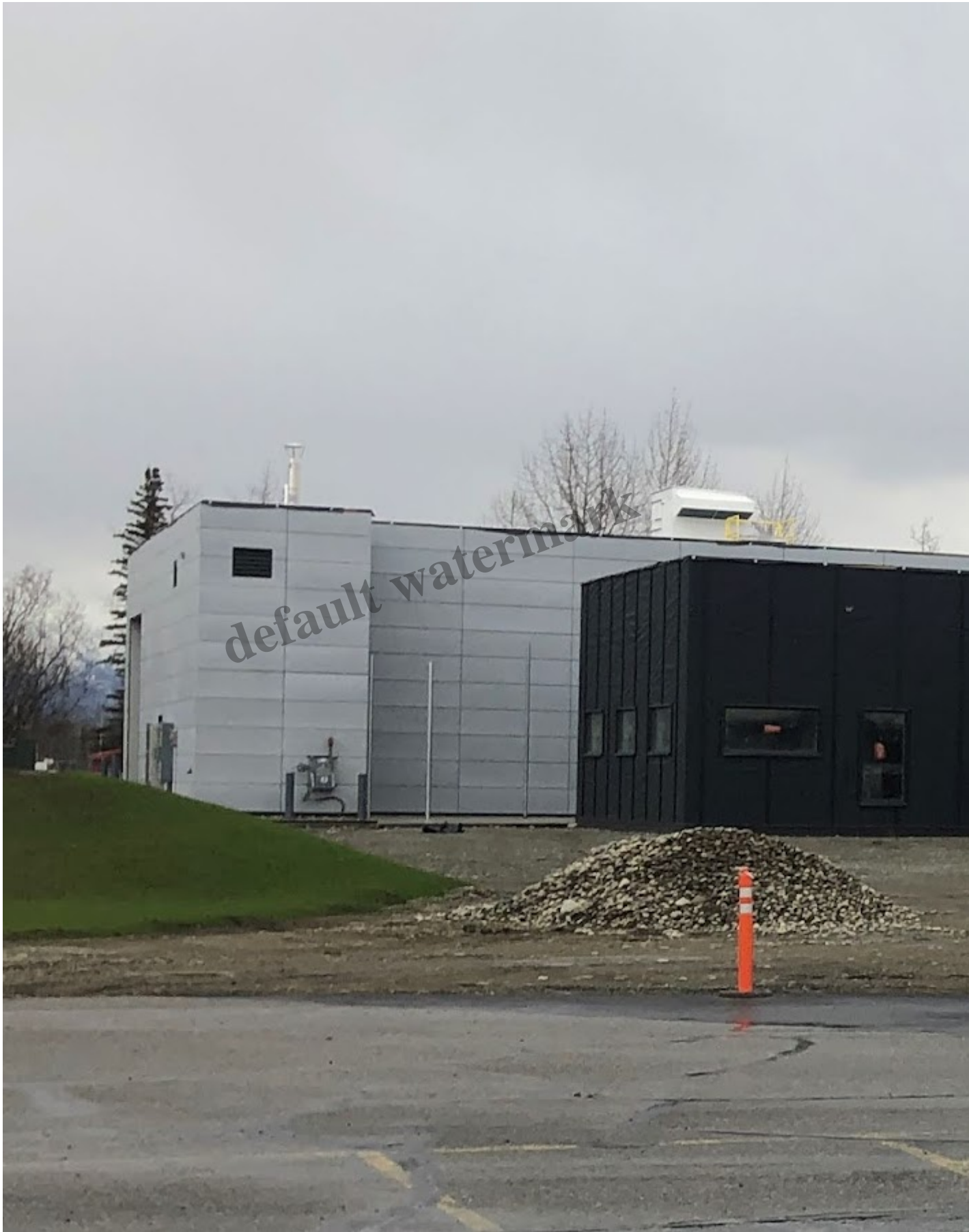
The new Wasilla Police station is under construction and expected to be completed ahead
