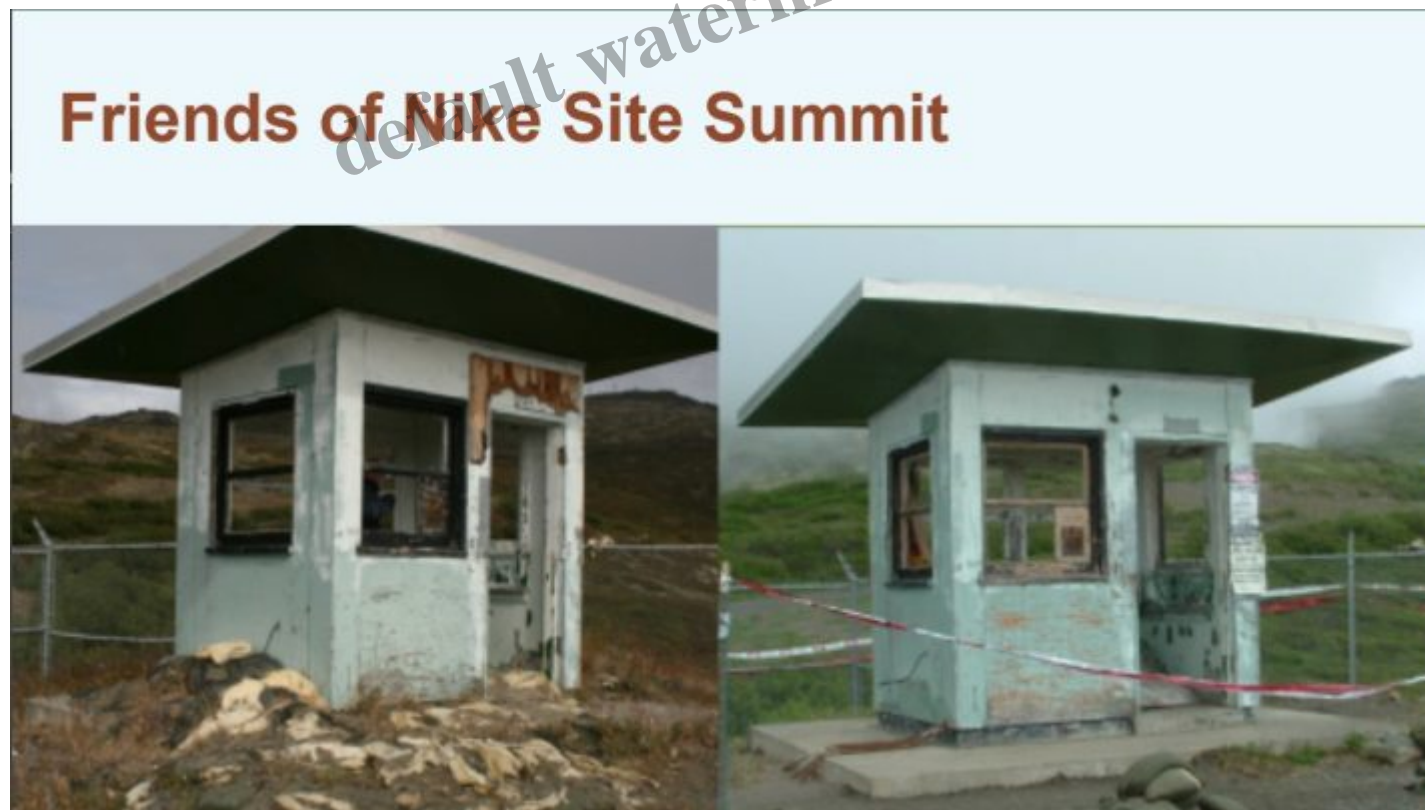
The guard shack renewal demonstrates how restoration is coming along at the Nike Site above Anchorage.
